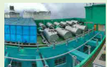
Renewable energy hot water system at FWH.
